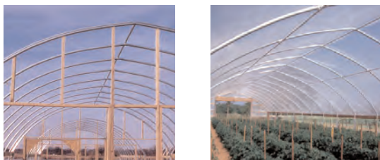
Figure 4. Purlins can number from one to four on a high tunnel.
