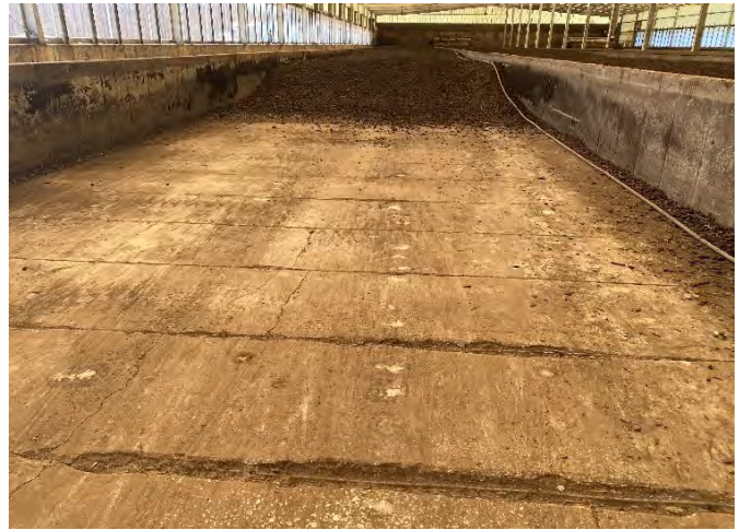
Figure 6. Air supply pipelines are installed at the bottom along the compost pit row and are not operating because the mixing vessel created enough aeration, and the aeration requires a lot of maintenance.
