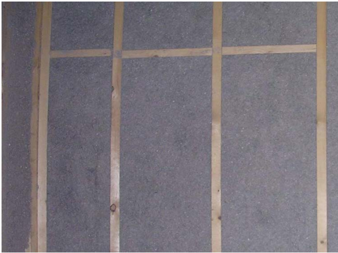
Figure 1. Blown-in cellulose insulation between wall studs.
