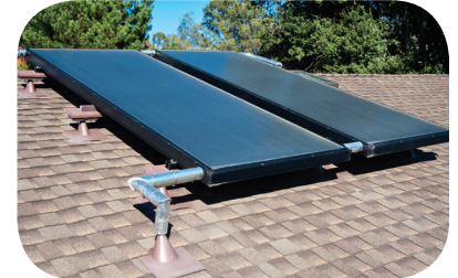
Roof-mounted solar hot water collectors.
