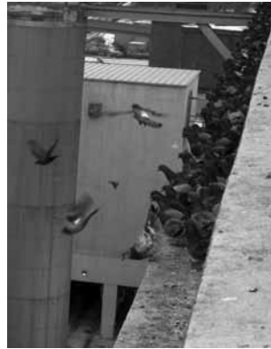
Figure 2. Pigeons can become a nuisance when large groups gather atop city buildings.
