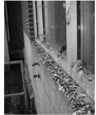
Figure 3. Pigeon droppings can be a health hazard if allowed to accumulate.
