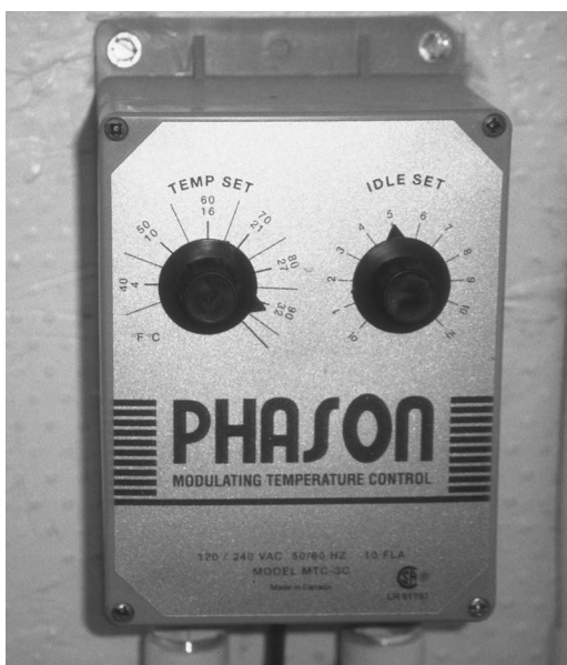
Figure 3. A modulating temperature control unit keeps a storage area at an ideal temperature.
