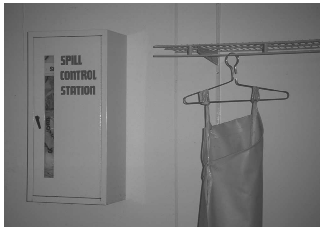
Figure 11. Provide tools and absorbant material to clean up spills.
