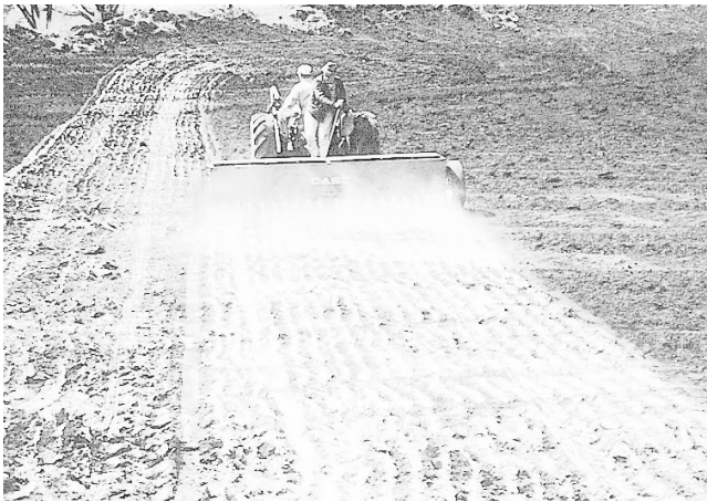
Figure 2. Dispersants such as sodium tripolyphosphate (STPP) may be spread and then disked into the soil before compaction to seal a pond bottom.
