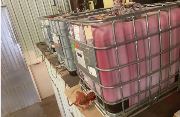
A system of three flow meters, allowing the accommodation of 210-gallon chemical totes.
