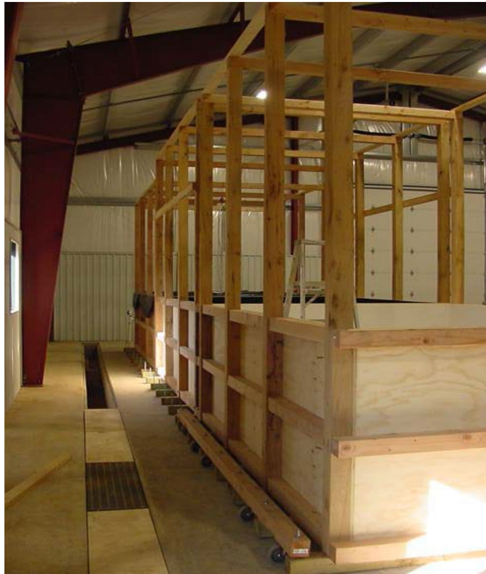
Prototype Raceways and Water Collection Sump
