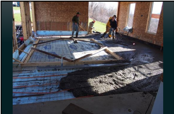
12x14 cooler-Insulation-Radiant Heat
