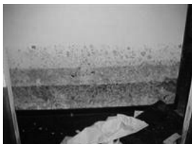
Mold on wall extends above flood level because the moisture wicked up the drywall.
