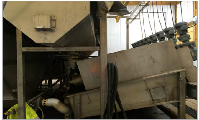
Figure 29b. Bank of MD presses dewatering DAF froth (side view).
