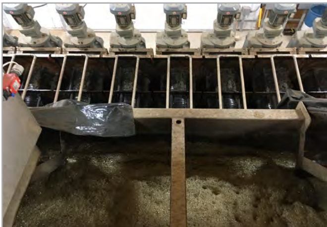
Figure 29a. Bank of MD presses dewatering DAF froth (front view).
