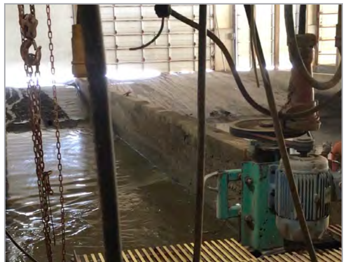
Figure 7. Digester surge pit, left; flush water pit, right.
