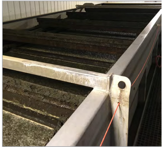
Figure 11. DAF with baffles pushing froth, or floating solids from aeration and flocculation processes.
