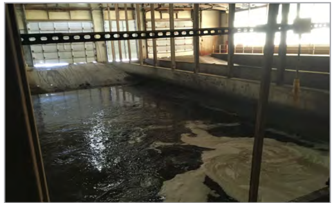
Figure 5. Flush water pit (raw manure pit in background).
