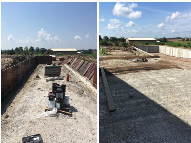
Figure 12. PPSB with concrete forms being set (left) and construction nearing completion (right).
