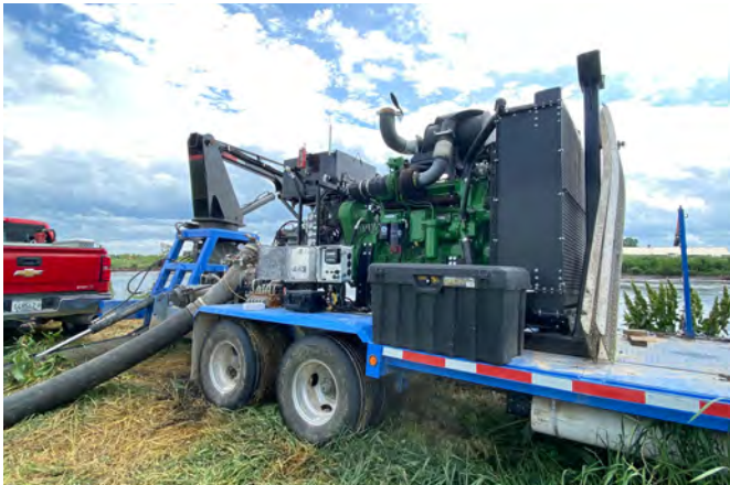
Figure 3. Primary lagoon pump (trailer mounted).
