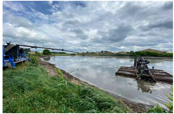
Figure 4. Boom intake and primary lagoon pump.
