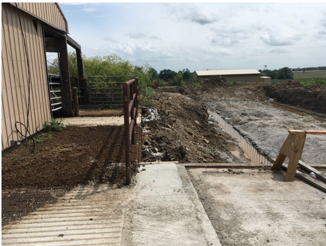
Figure 11. Early construction of the PPSB with flush trough and old drying pad.
