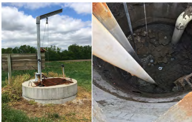
Figure 3. Lift station located next to the pig barns showing a crank system for pump maintenance and manhole steps.
