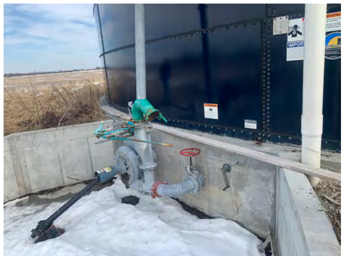
Figure 7. Centrifugal pump on a slurry tank with the valves, for agitation and pumping out the effluent.
